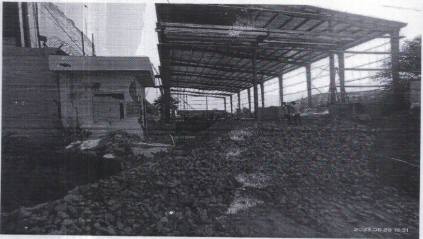
Plot No. F-50, G-51, EPIP, RIICO Industrial Area, Neemrana, Rajasthan (Proposed Project-1)
